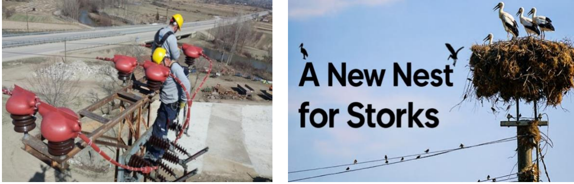
Figure 3. Insulation measures and a safe nesting platform to reduce electrocution risk
